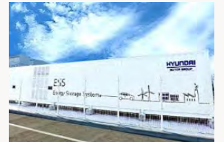
2MWh ESS at Ulsan plant
