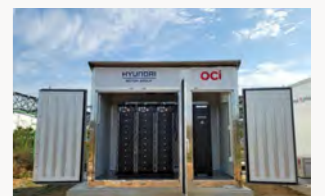
300kWh commercial ESS at the OCI Plant
